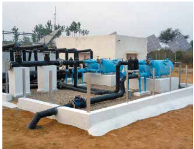
328 kW (245 hp) Solar Pumping Station
