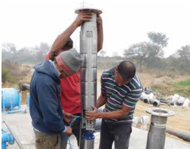
Solar Pump Assembly
